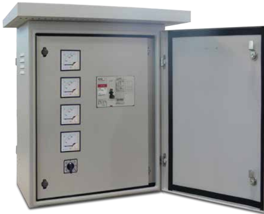
LV Board With Components
